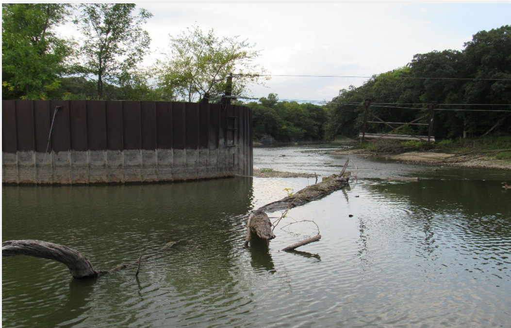
Figure 27 – Upstream, Spillway 3: Timber Debris Accumulation
