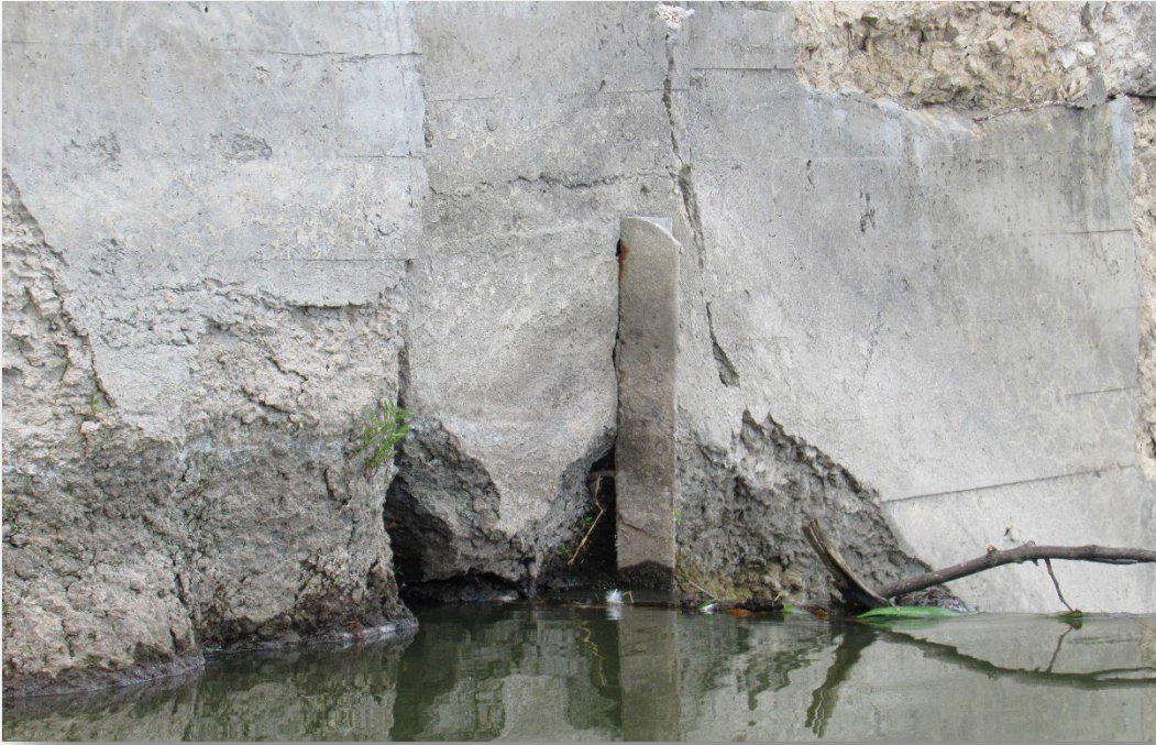
Figure 14 – Upstream, Control Gates West Pier: Spalling and Vertical Crack
