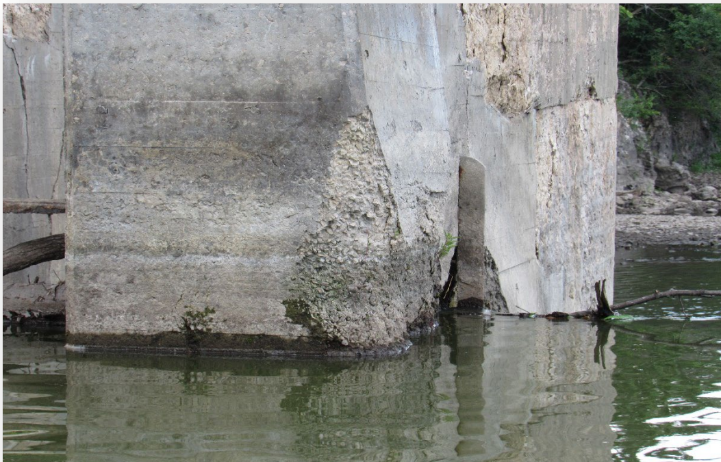
Figure 13 – Upstream, Control Gates West Pier: Scaling
