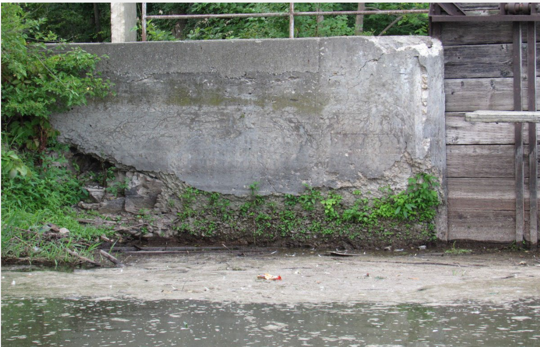
Figure 3 – Upstream, Eastern Bypass: Scaling and Spalling
