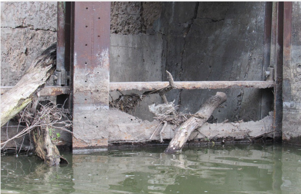
Figure 11 – Upstream, Control Gates: Holes in Gate
