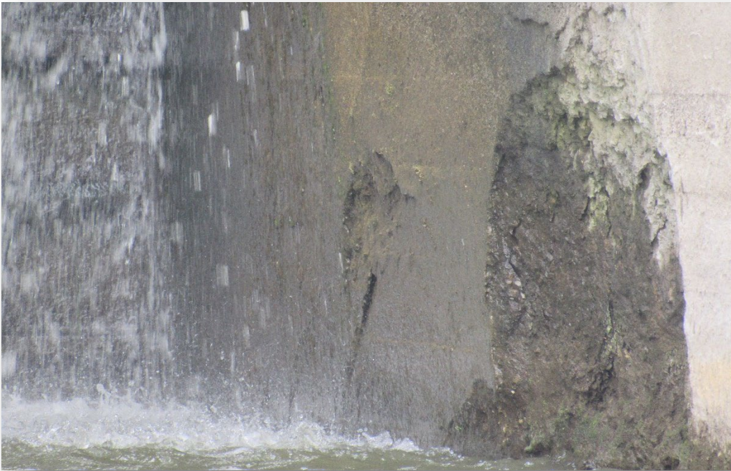
Figure 44 – Downstream, Control Gates: Spalling
