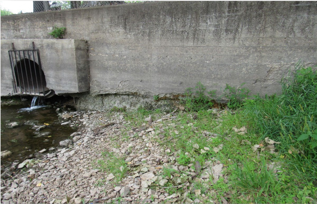
Figure 36 – Downstream, East Wingwall: Band of Scaling
