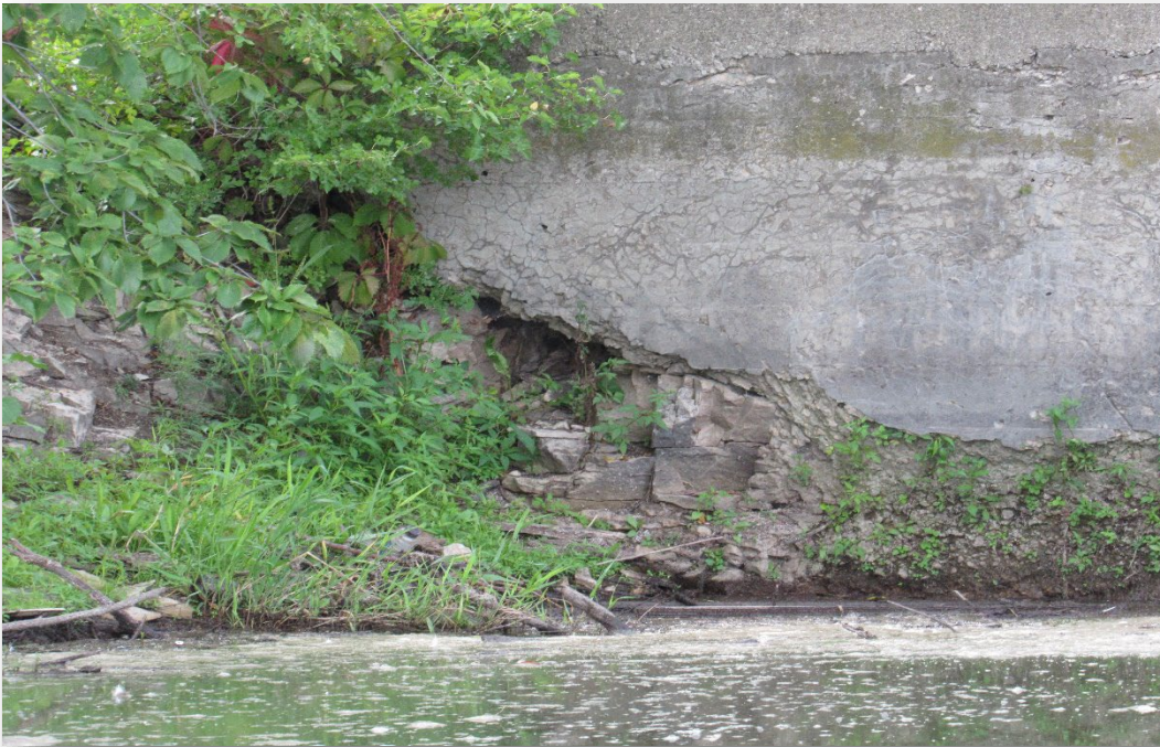
Figure 4 – Upstream, Eastern Bypass: Spalling
