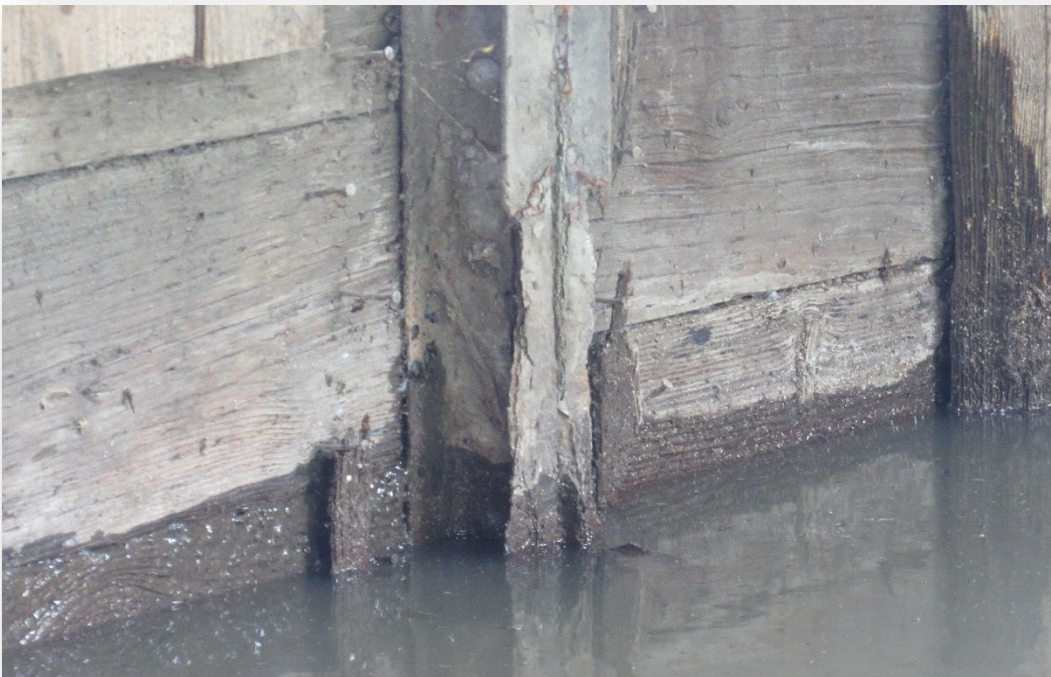
Figure 35 – Downstream, Eastern Bypass Vertical Support: Delamination
