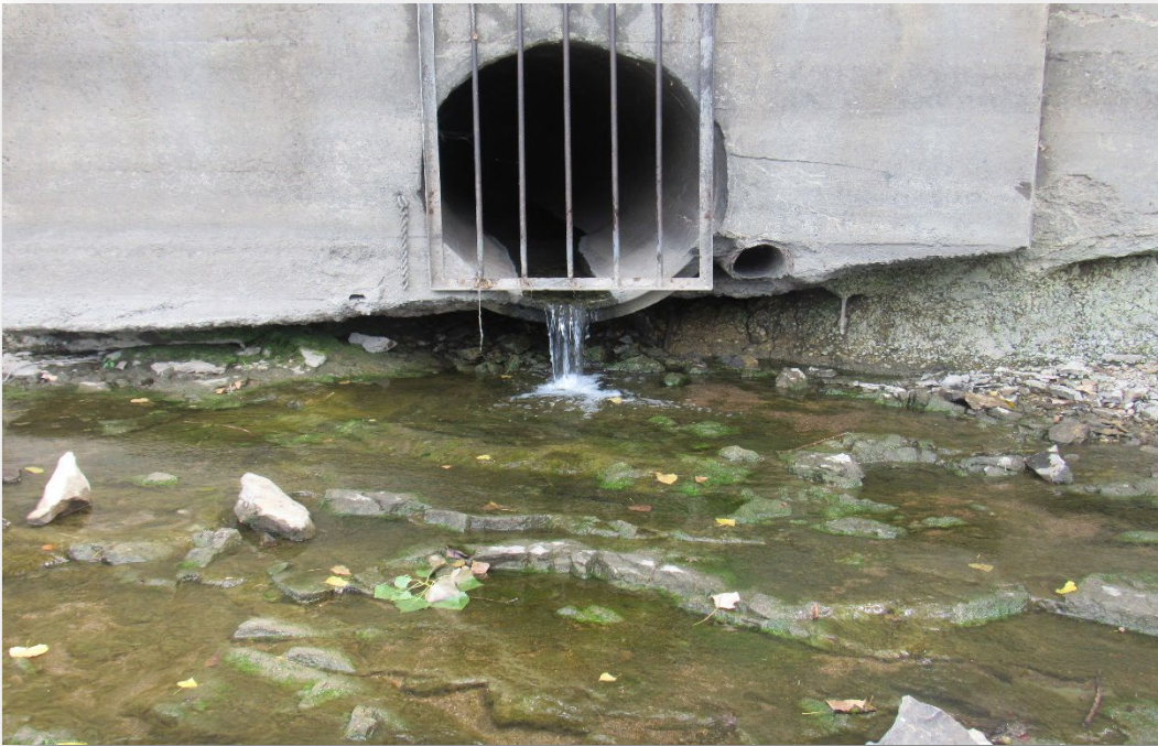
Figure 38 – Downstream, East Wingwall Drainpipe: Undermining
