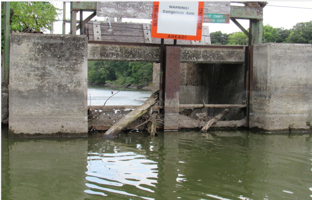
Figure 12 – Upstream, Control Gates: Condition of Gates and Timber Debris
