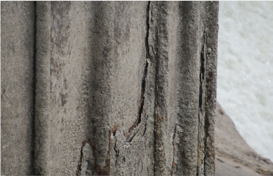
Figure 52 – Downstream, Cell Section: Delamination
