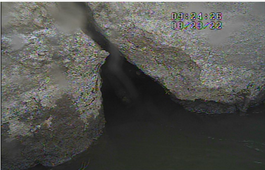
Figure 59 – Upstream, Control Gate West Pier: Spalling
