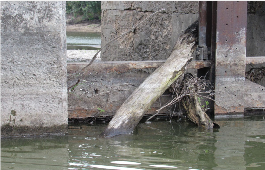
Figure 10 – Upstream, Control Gates: Timber Debris
