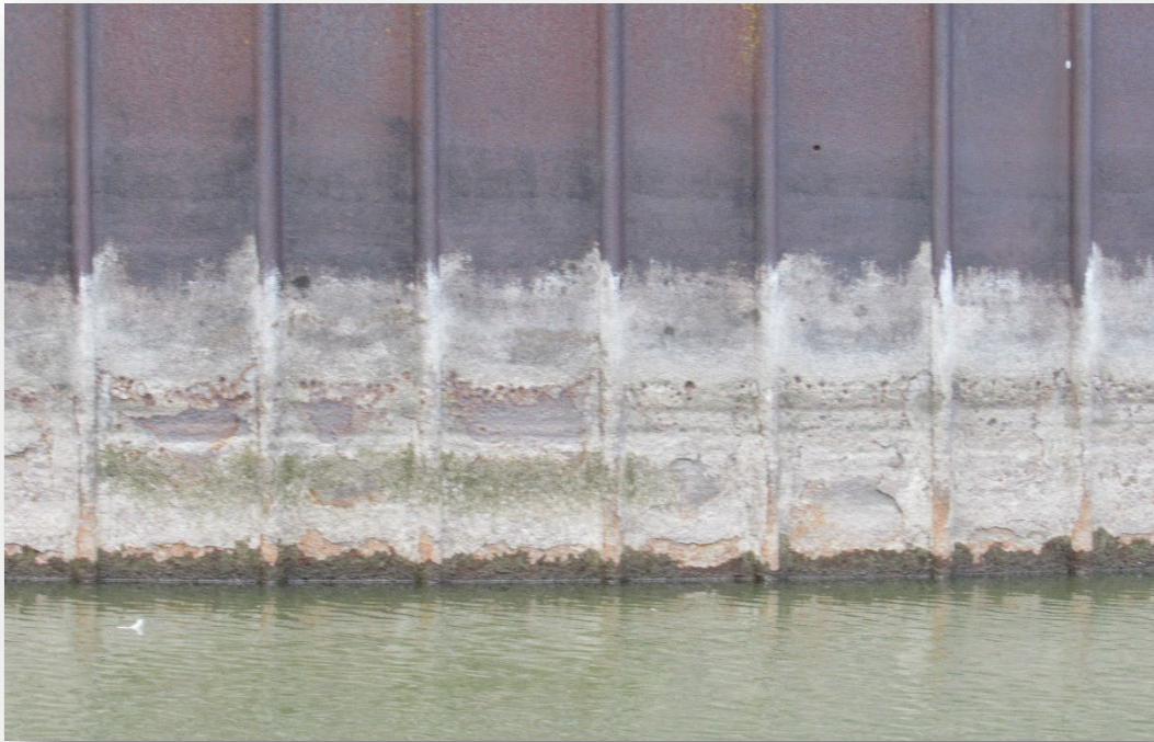
Figure 26 – Upstream, Cell Section: Typical Rust and Delamination
