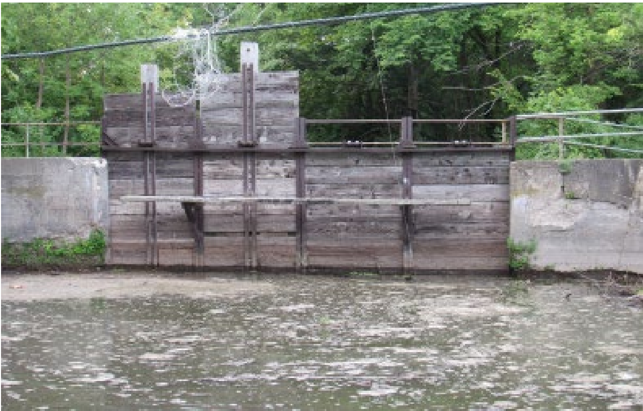
Current condition of the vertical lift gate with the old mill-race gate also shown.
