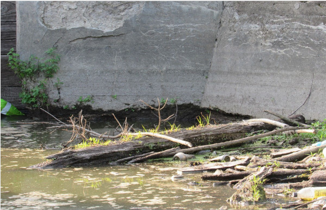
Figure 6 – Upstream, Eastern Bypass: Freeze/Thaw Band
