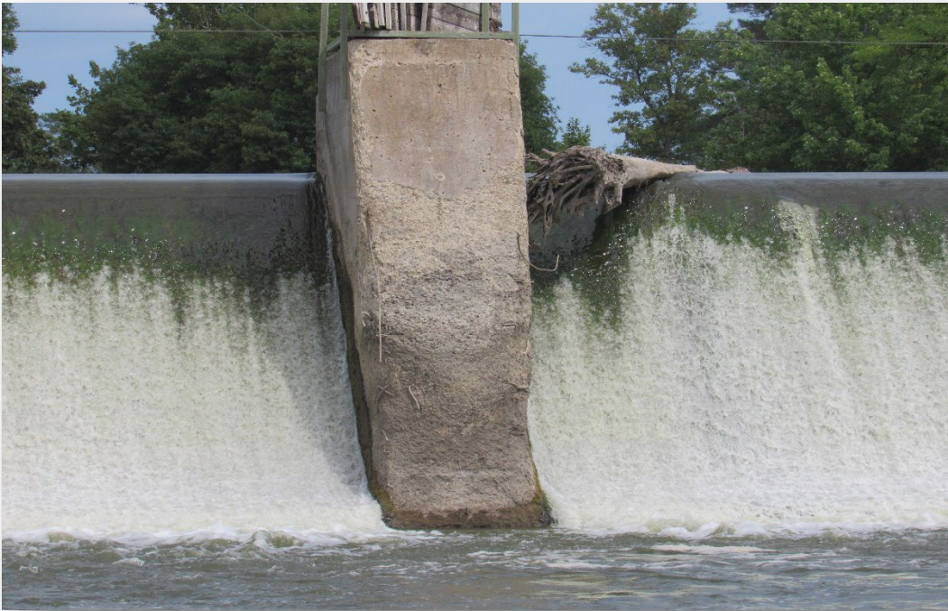
Figure 50 – Downstream, Spillway Center Pier: Heavy Scaling and Exposed Rebar
