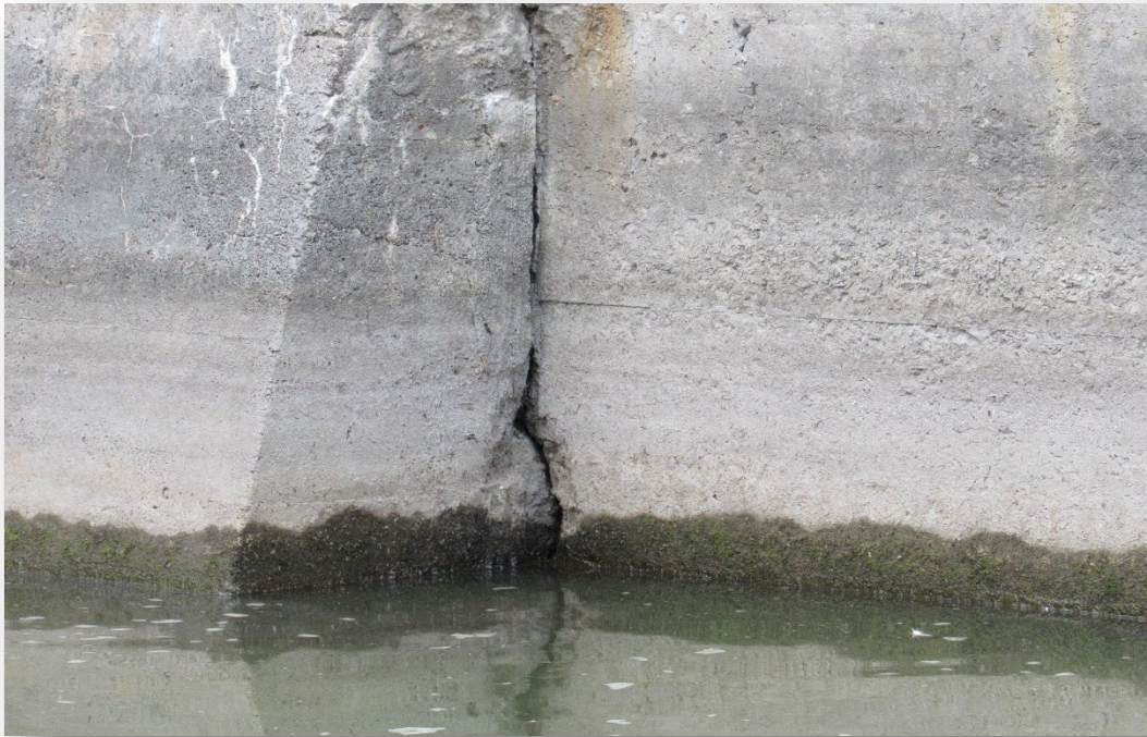
Figure 8 – Upstream, Control Gates East Pier: Vertical Crack
